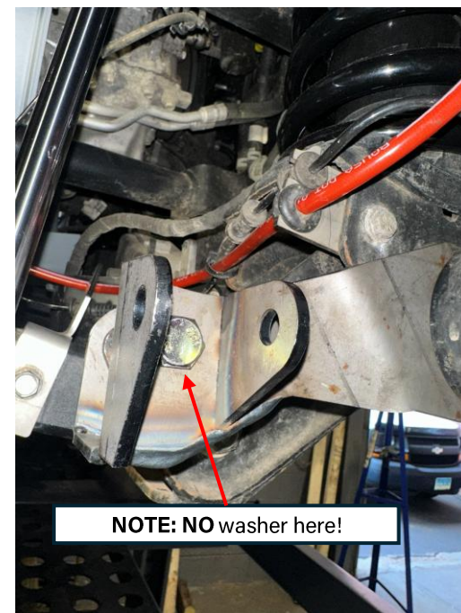
Figure 7: No washer at bolt head
