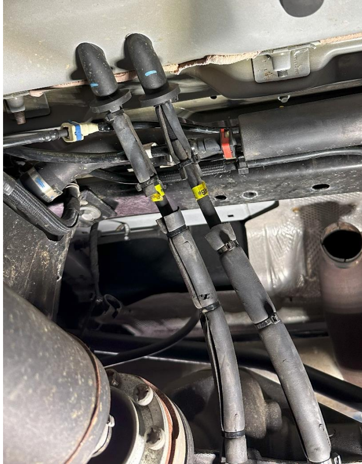
Figure 3: Emergency brake cable housings pulled out from above cross member and rerouted below the fuel line
