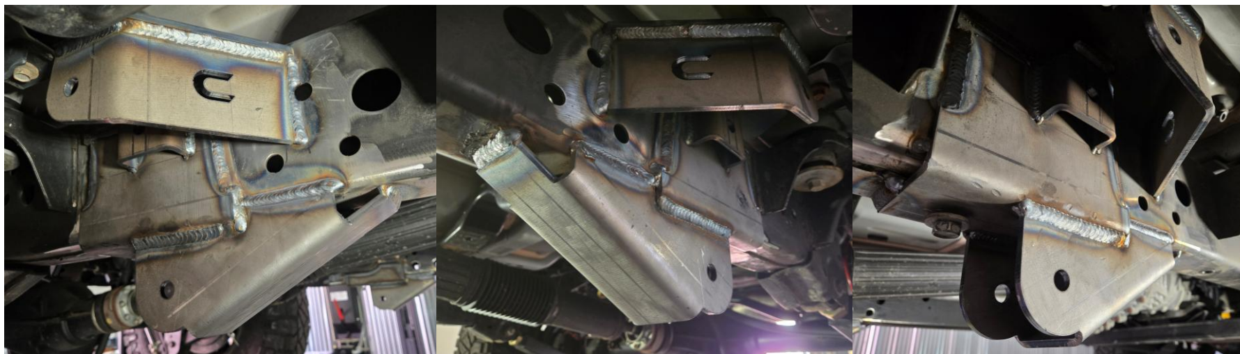
Figure 16: Bracket welded along the contact edge points to frame rail
