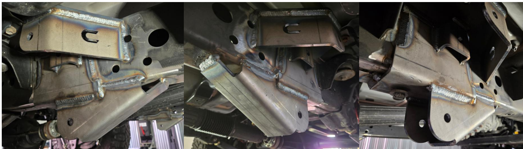
Figure 27: Bracket welded along the contact edge points to frame rail
